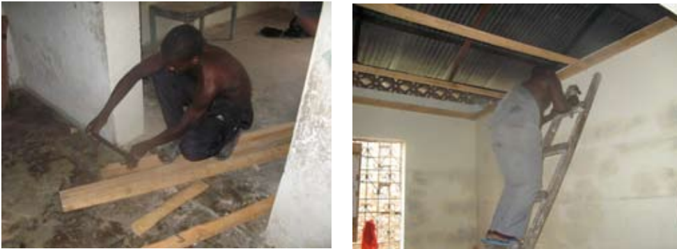
Our office in Mombasa is being restored by former street boys. They are now educated carpenters.
